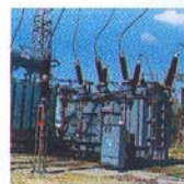
Transmission & Distribution Substation
